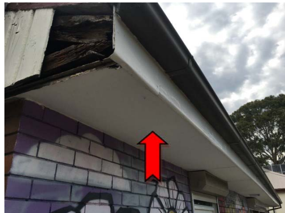
Photo 4. Exterior, throughout, eaves – asbestos-containing fibre cement sheeting.
