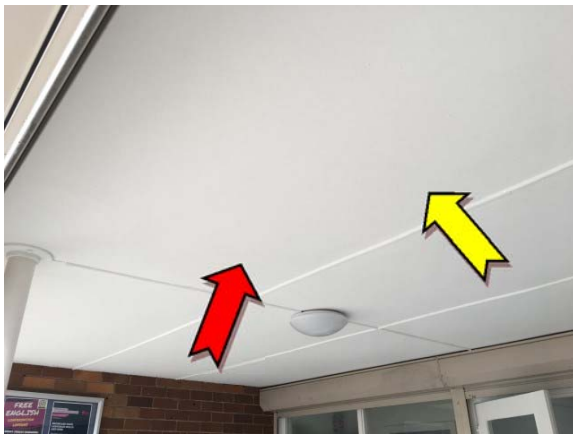
Photo 3. Exterior, courtyard entrance, awning – asbestos-containing fibre cement sheeting and suspected lead-containing white upper paint systems.
