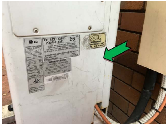
Photo 10. Exterior, north-west elevation, air conditioning unit – suspected non ODS-containing unknown refrigerant.
