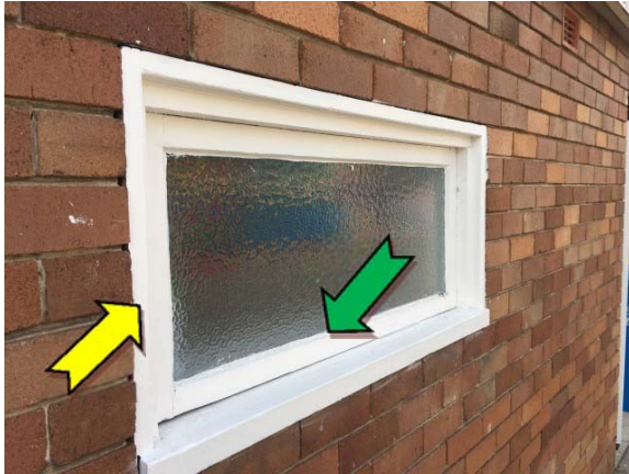
Photo 1. Exterior, throughout, window frames – non asbestos-containing window caulking and suspected lead-containing white upper paint system.
